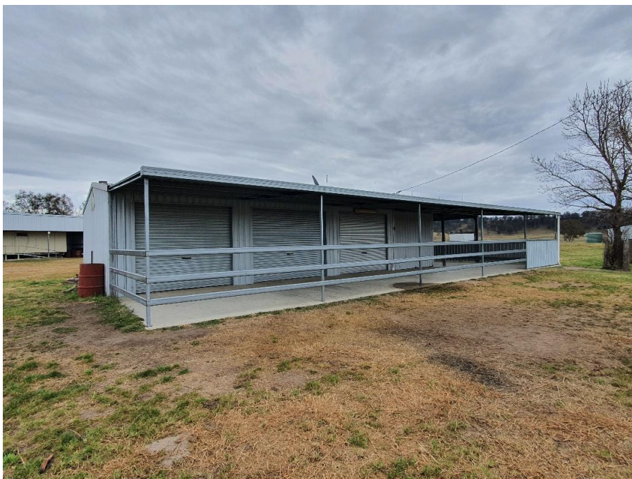
Canteen and Social area Condition Rating: 2
