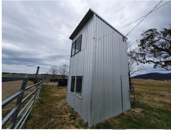
Secretary and Commenter's box Condition Rating: 3
